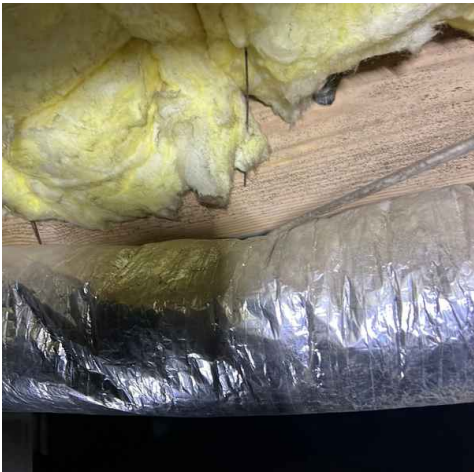
Fungi in crawlspace multi locations
