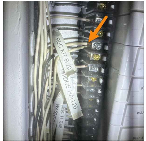
Main house panel
