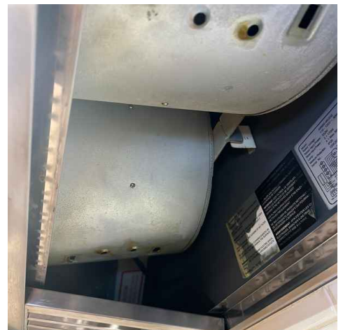
Vent hood gease on motors
