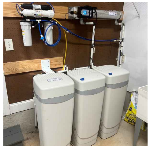
Component not inspected-Garage utility closet
