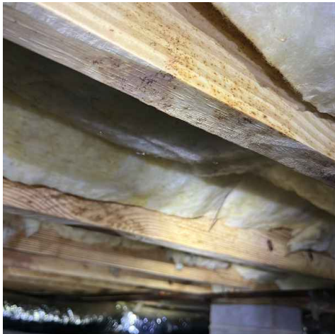
Fungi on floor joists in CS
