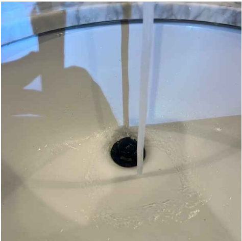
Drain stopper malfunctioning
