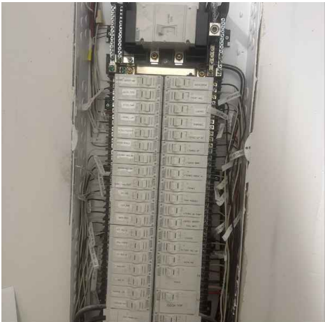
Garage main panel
