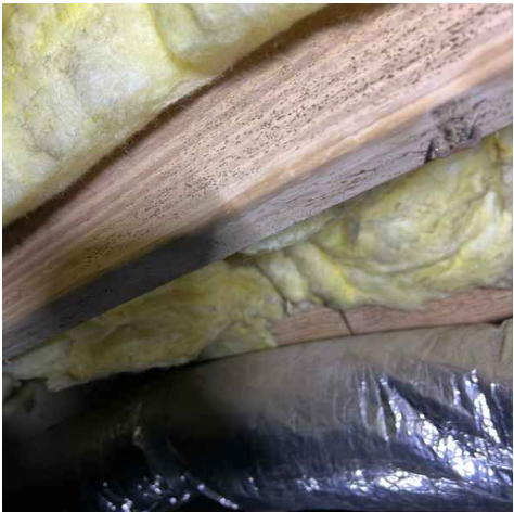
Fungi in crawlspace multi locations
