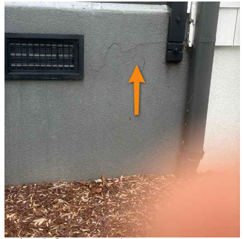
Below left rear porch
