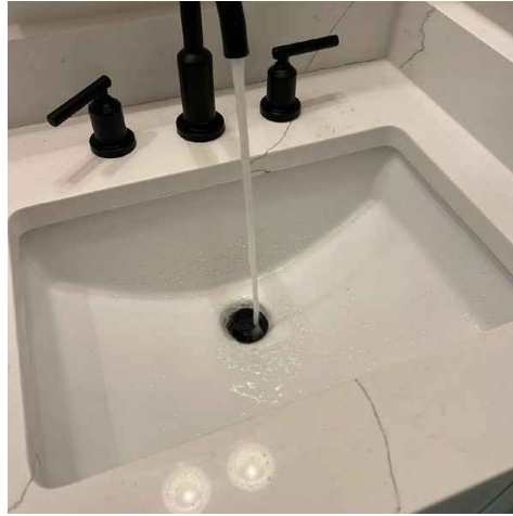
Right sink drain stopper
