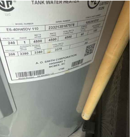
Water Heater Data- Apartment / Garage
