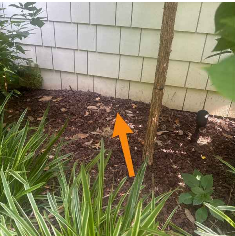
Garage front left below window
