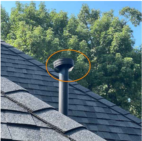
Second floor gas heater vent cap
