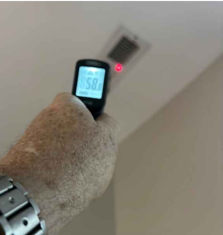
Second floor AC temp- House
