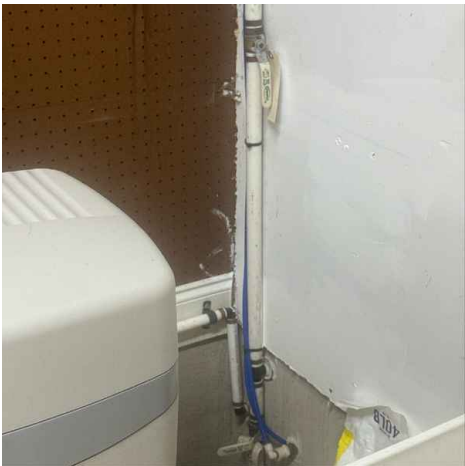
Main water shut off valve- Garage utility closet
