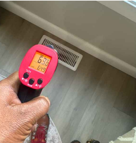
Second floor AC temp- Apartment
