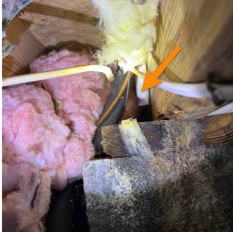
Drain line not connected Middle Front in CS
