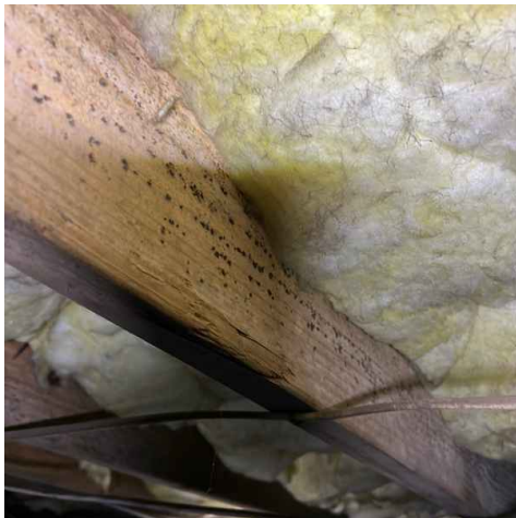
Fungi in crawlspace multi locations
