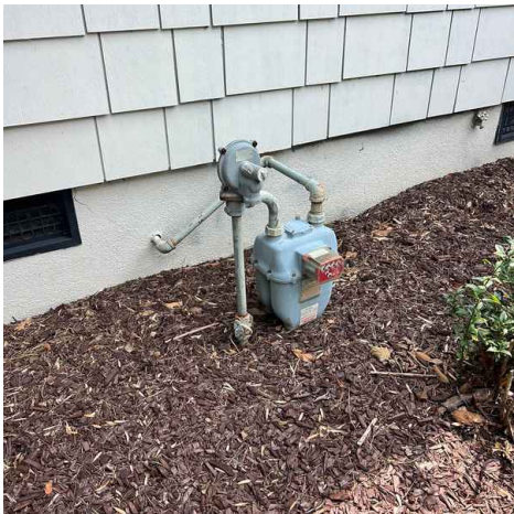
Gas meter left side
