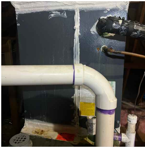
Second floor AC Indoor coil unit- Attic
