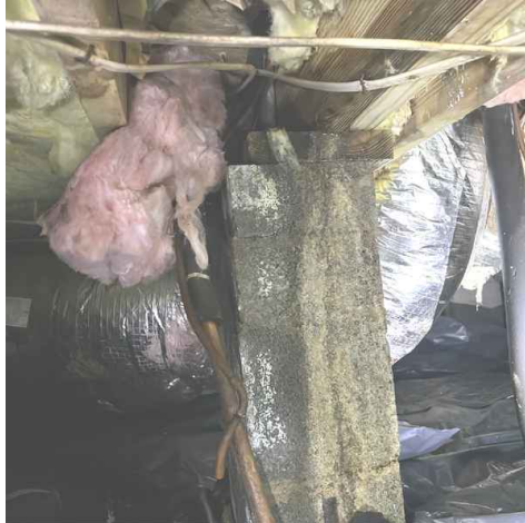
Drain line not connected causing wet blocks
