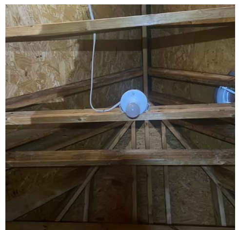
Attic lights out
