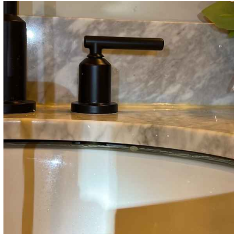
Sink disconnected from countertop
