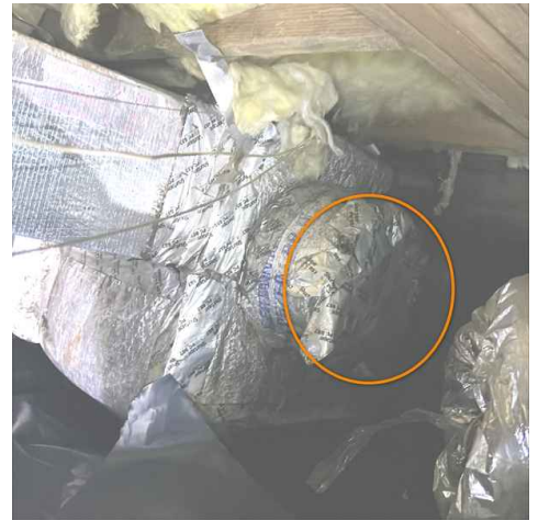
Distribution box in CS-Middle front
