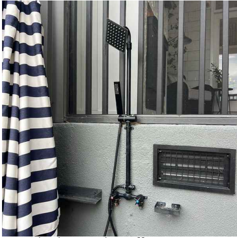
Outside shower shut off
