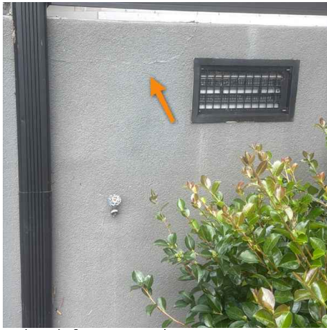
Below left rear porch
