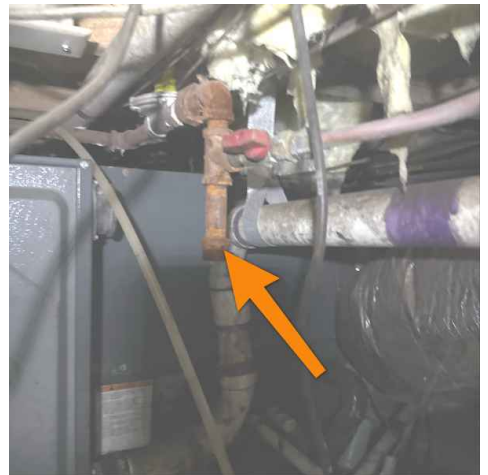
Gas line at CS heating unit
