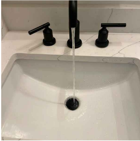
Left sink drain stopper
