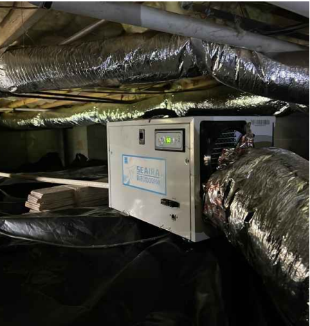
Dehumidifier in CS
