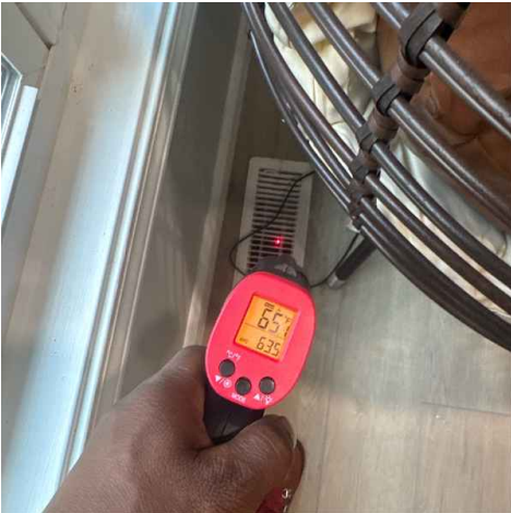
Second floor AC temp- Apartment
